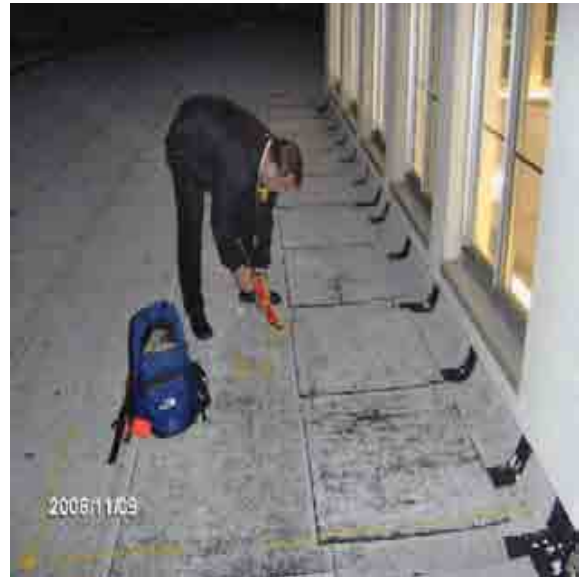
Roof 1-11 A hole was discovered in the roof membrane and was temporarily repaired by Roof Solutions.
