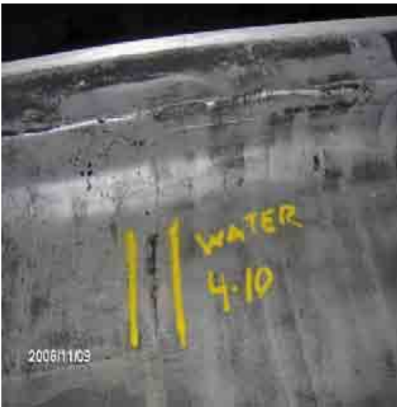
Roof 4-10 Another location with water present under the membrane.
