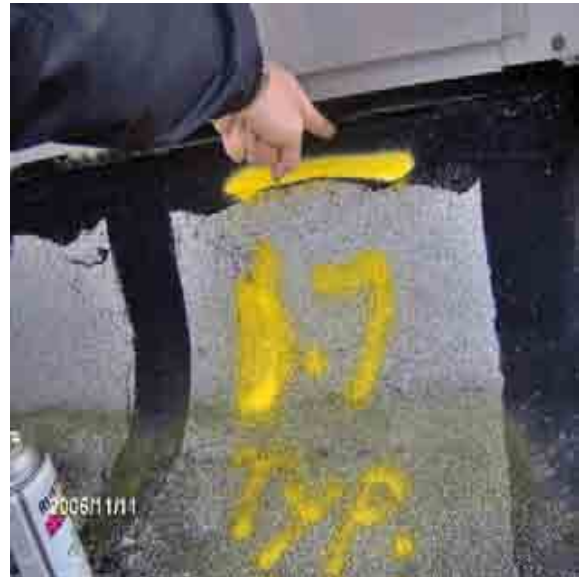
Roof 1-7 The base flashing needs to be properly terminated and have counter flashing installed.
