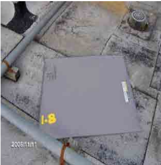
Roof 1-8 Metal panels and debris can become airborne and cause damage to the roof or pedestrians.
