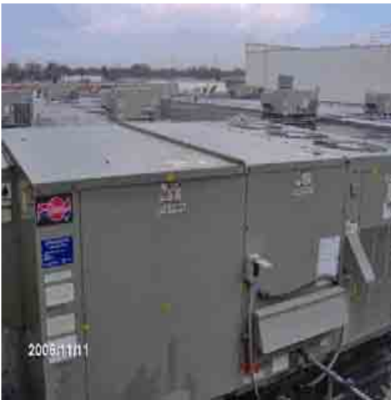
Roof 3-1 HVAC units. These units have failing seals, missing fasteners and screw.
