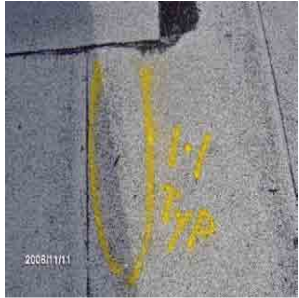
Roof 1-1 Small blisters are typical and need to be monitored.
