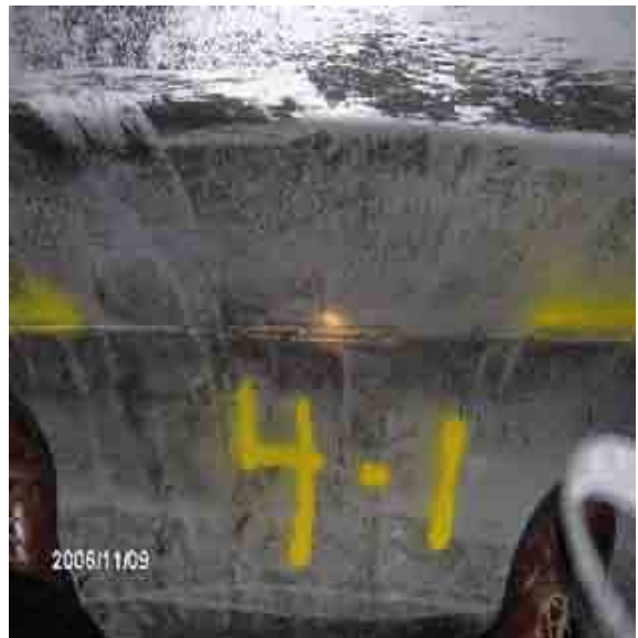
Roof 4-1 Wall flashings are splitting open.
