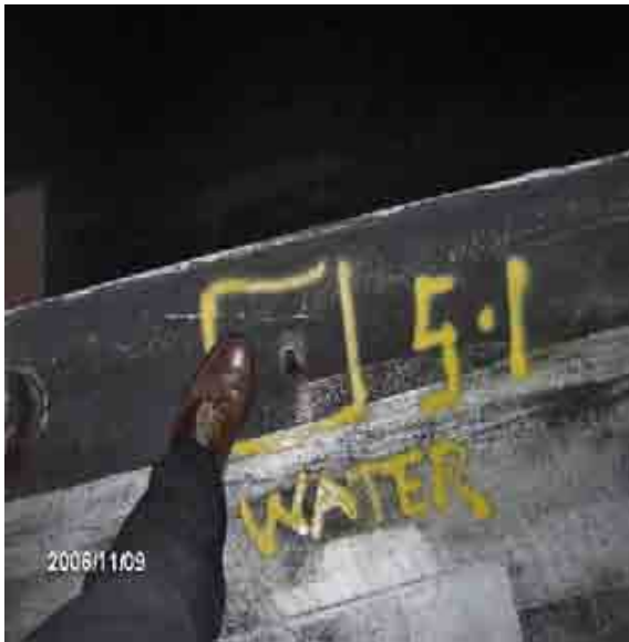
Roof 5-1 Water was found along the edge at this hole in the membrane.
