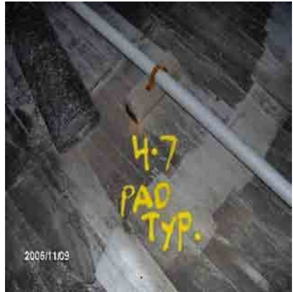
Roof 4-7 Protection pads need to be installed at all locations of wood sleepers.
