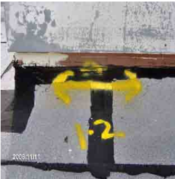
Roof 1-2 The top of the flashing are exposed. Install termination bar and slip metal counter flashing.
