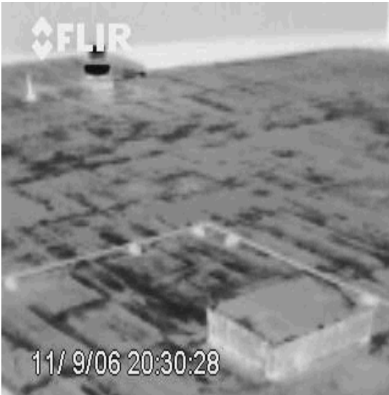
Roof 5 Infra-red overview of Roof section 5. No wet areas were observed.
