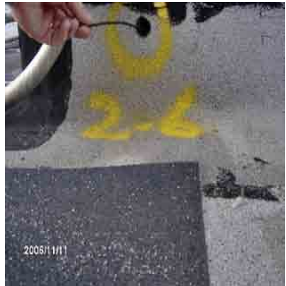
Roof 2-6 Improper flashing. The hole is open.
