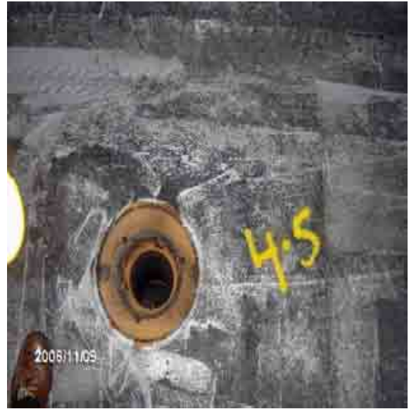
Roof 4-5 Drain strainers should be installed to prevent debris from blocking the drain lines.
