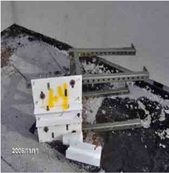
Roof 1-4 Metal debris will puncture the membrane.
