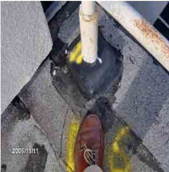
Roof 1-6 The penetration pockets are all in poor condition and should be topped off and a hood added.
