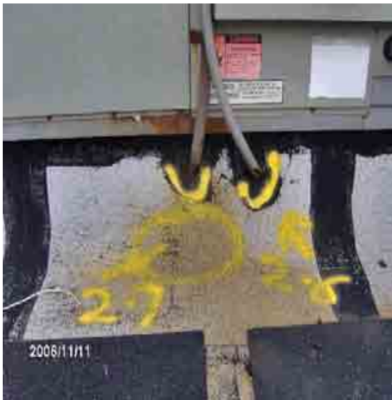
Roof 2-7 Open conduit flashing. Conduits should not be installed through the side of the curb wall.
