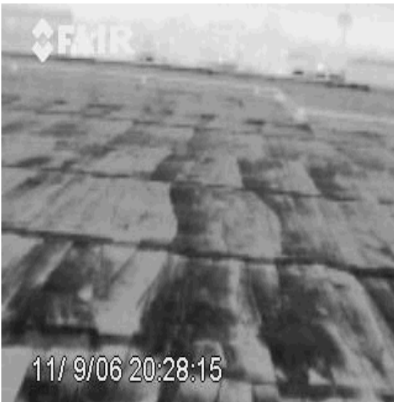
Roof 4 The infra-red overview of this roof section showed the rear one third of the roof to be wet.
