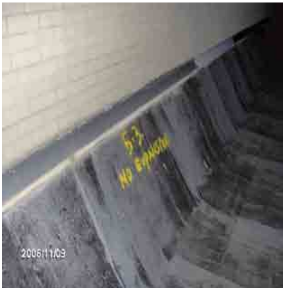
Roof 5-3 An expansion joint should have been installed to accommodate the movement of the two separate buildings.
