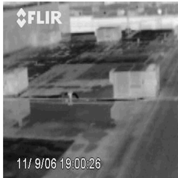
Roof 3-6 An infra-red overview of Roof 3. The amount of ponding and patches made this roof section difficult to scan. Cores showed the roof to be wet.
