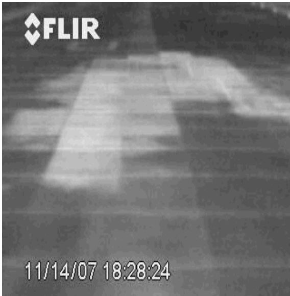
Roof 1-16 The right angles are created as water spills over into an adjacent insulation board.
