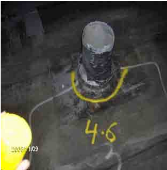
Roof 4-6 This flashing is open. It was marked as wet in a previous scan.
