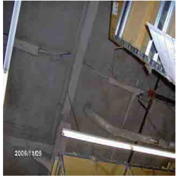
Roof 5 Deck underside. The fireproofing was spray applied to a metal mesh attached to the deck underside.
