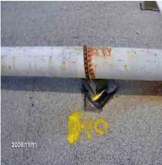
Roof 1-10 This wood block has damaged the membrane.
