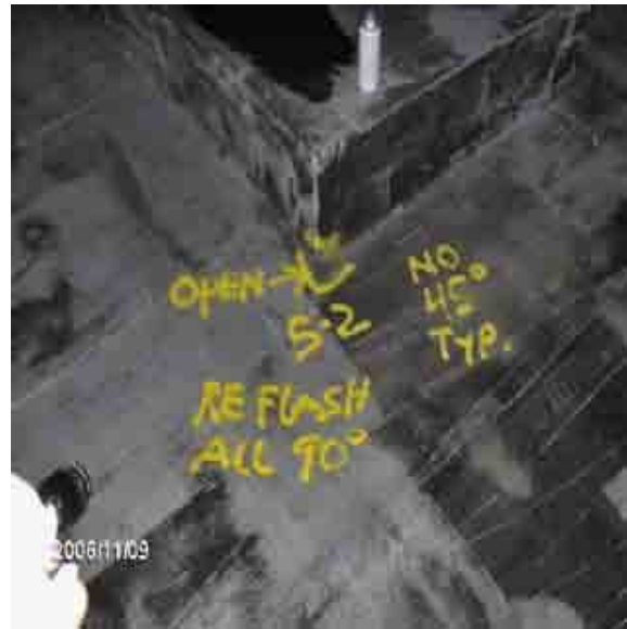
Roof 5-2 Reflash all 90 degree angles on the penetrations.
