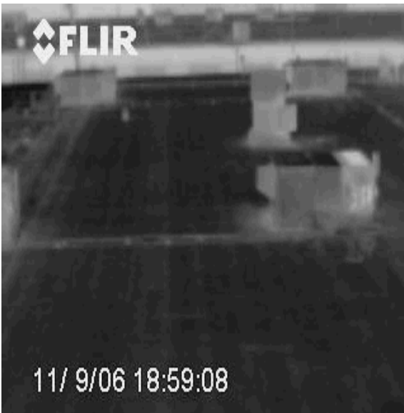
Roof 2-11 This is an infra-red overview of Roof 2. No anomalies were discovered.
