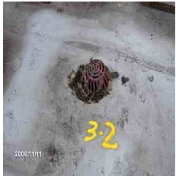
Roof 3-2 Drain strainer not attached. Clean debris.
