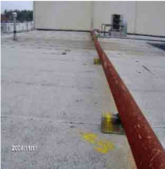
Roof 2-3 All the wood blocking should have new bands installed to secure the blocking from moving.
