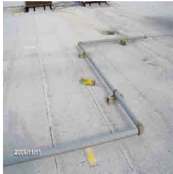
Roof 1-9 Wood blocking should be secured to the pipe. Protection pads should be installed under all wood blocking.
