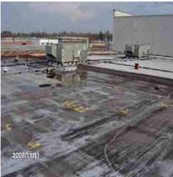
Roof 3-5 Area of bad deck. An area of ~ 18' x 18' is of serious concern. This should be cordoned off.
