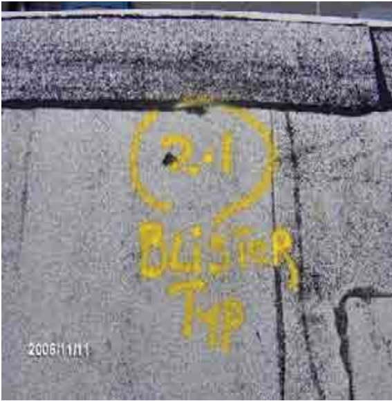
Roof 2-1 Blister was observed and marked. These should be monitored.
