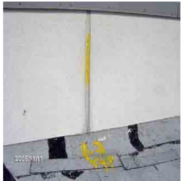
Roof 1-3 The wall joints are deteriorated.
