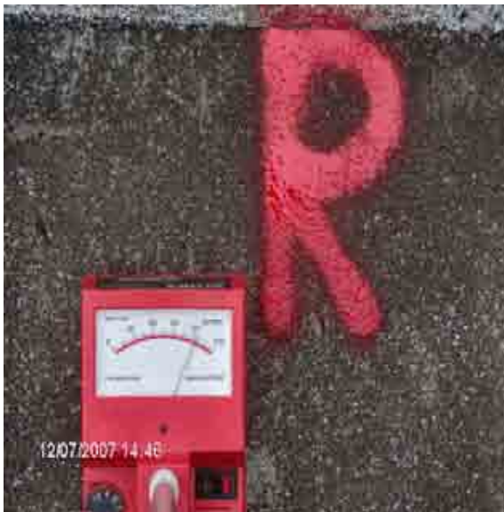
Roof 1-18 Moisture was registered on the Tramex/Capacitance Meter.
