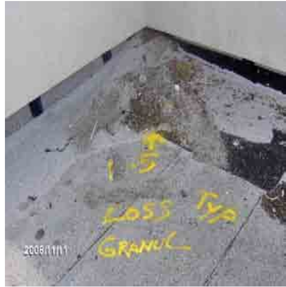
Roof 1-5 The pile of granules is an indication of the extensive granular loss exhibited on this roof. This situation should be monitored.
