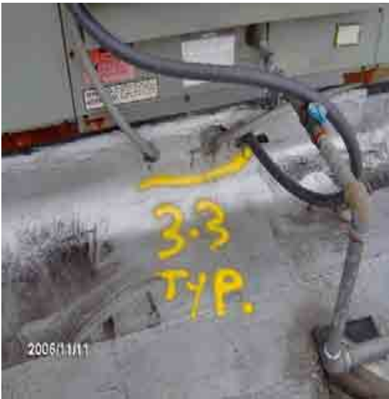
Roof 3-3 Improper conduit flashing.
