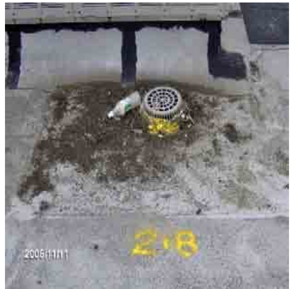
Roof 2-8 Clean drains periodically.
