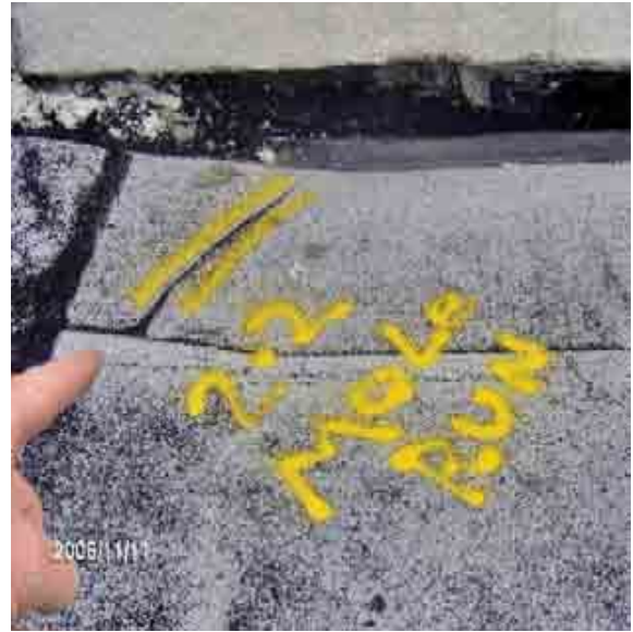
Roof 2-2 This mole run should be cut open and patched.
