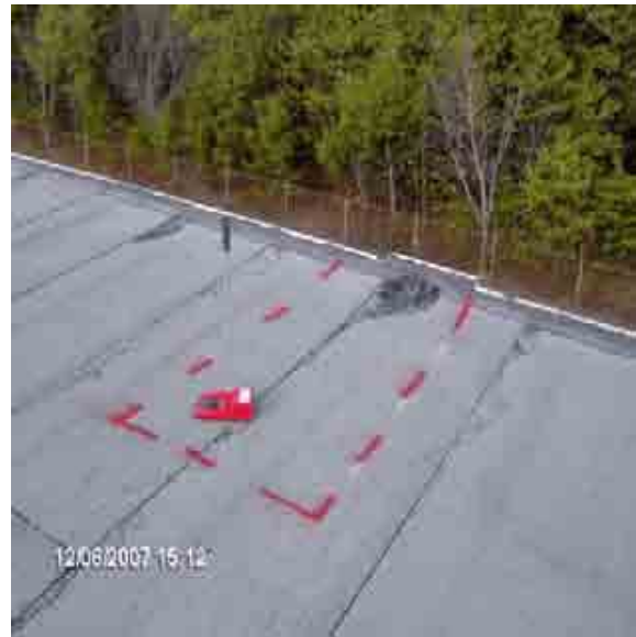
Roof 1-17 The capacitance meter registered moisture in the insulation.
