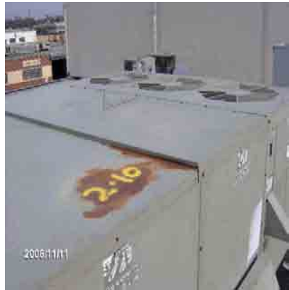
Roof 2-10 The seals are failing. These types of conditions should be monitored.
