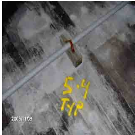
Roof 5-4 Secure all wood blocking with a band and add a protection pad beneath.
